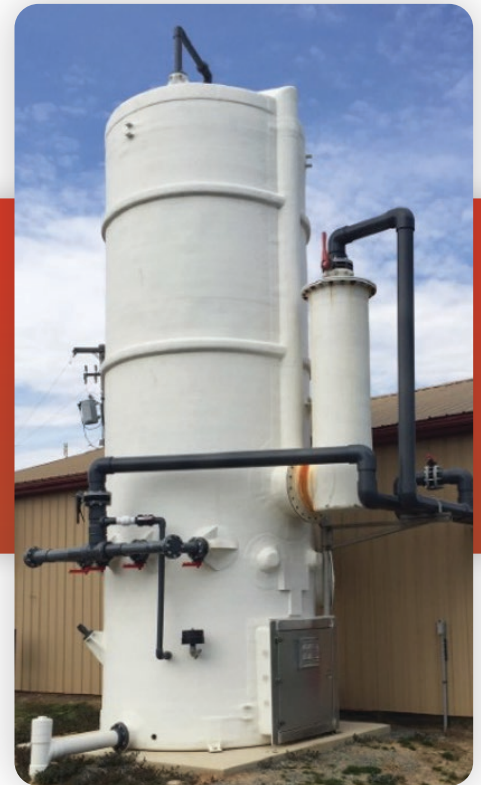
Figure 2. Methane gas scrubbing equipment improves the system's longevity.
