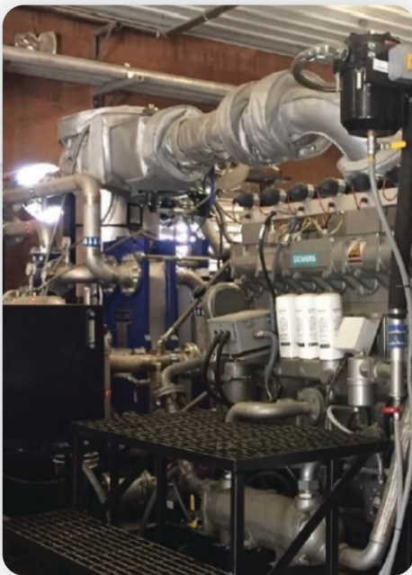
Figure 3. A 335-kW engine generates power and heat for the dairy farm from the farm's waste.
